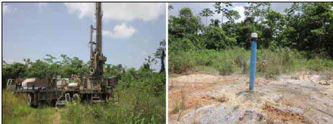
Fig. 19 Photo documentation from drilling of the HGE-1 borehole in Deep River Forest Reserve.
